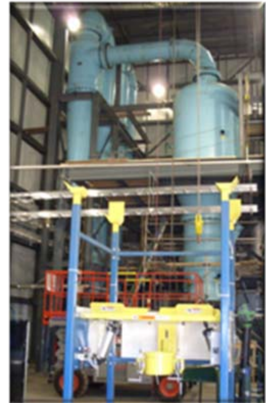
Gasifier and Gas Conditioning Equipment - August 2008
